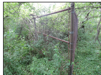
Maintenance yard fence blocks equipment access to north side of stream
