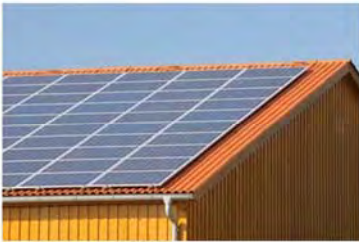
▲ Solar Tin Roof
