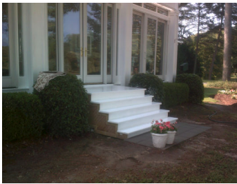
This stairway lack railings.
