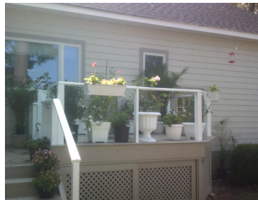
This porch lacks balusters.
