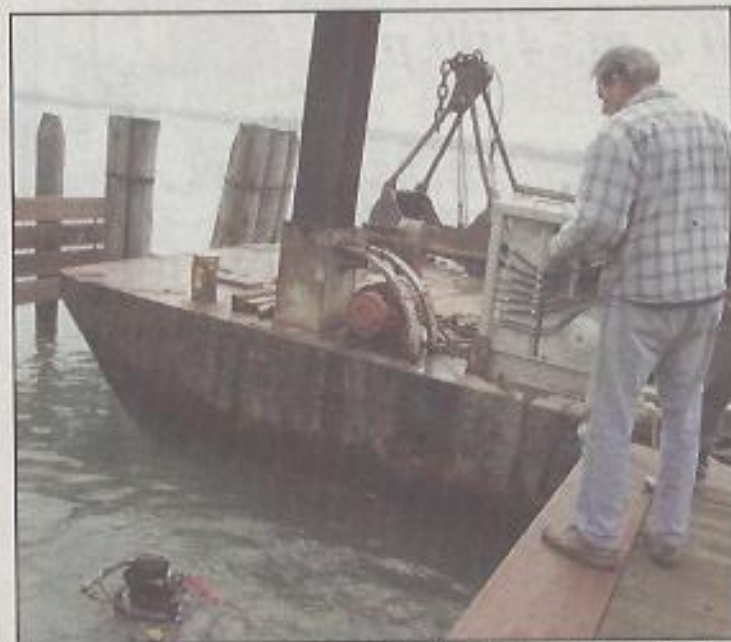
Diver Kolet and Captain Bud coordinate their plans for removing the broken pylon.
