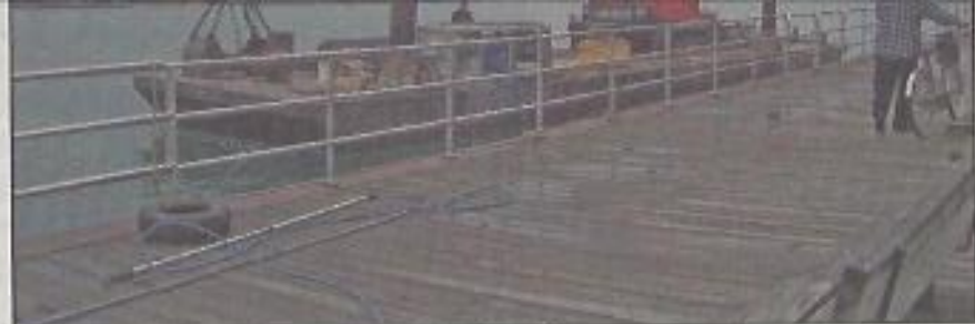
The crane on the barge is used to remove the broken pylon.
