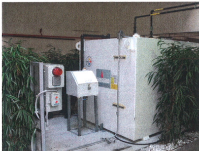
Generator Fuel Tank at Baptist Hospital
