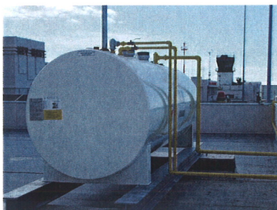
Generator Fuel Tank, Generator and Day Tank at Key West Airport
