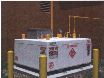
Emergency Generator Tank at Embassy Suites Hotel
