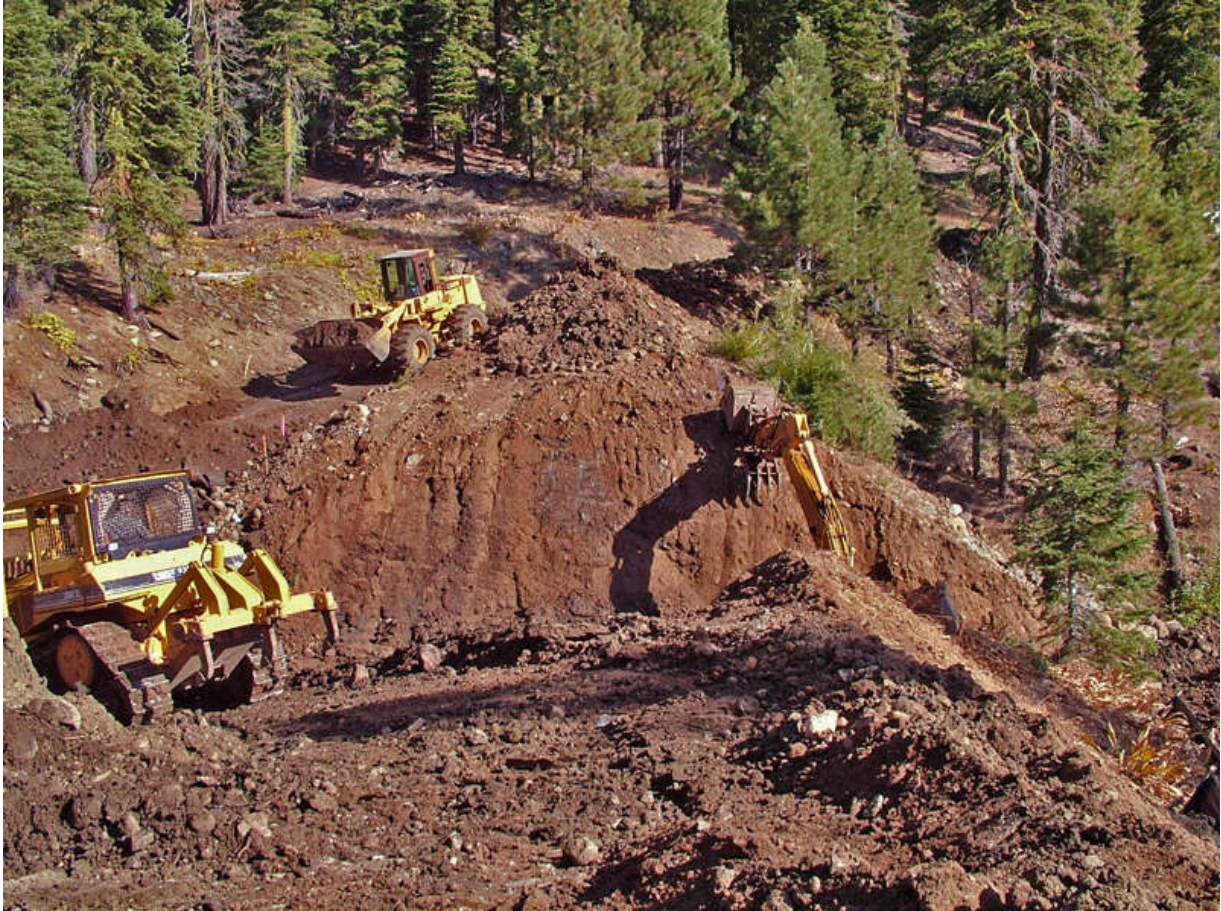
Photo 13. Remediation and obliteration of existing forest roads, can alleviate road impacts on watershed functions over time, contributing to the recovery of hydrologic flow routing, erosion, sediment delivery, and water quality. Plumas National Forest. Photo by C. Frissell.
