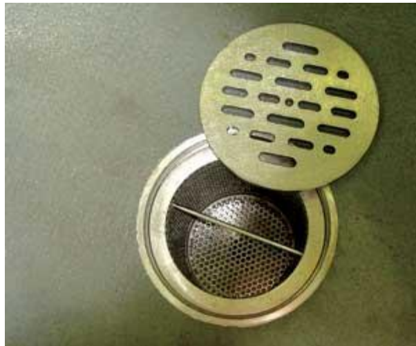
Figure 4. To make it even more difficult for bacteria to gain a foothold in the Overhill plant, much of the equipment and materials-including the drains-are made from stainless steel. Photo courtesy of Overhill Farms.
