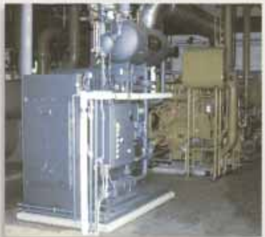
WATER PURIFICATION PLANT , Burlington, Ontario Model ESG1-A12D18CSS Recovering Btu from a Caterpillar 3516, 800kW natural gas engine. Reducing 2,382 SCFM from 770°F to 344°F. Delivering 1,277 pph steam @ 130 PSI operating (150 PSIG design).
