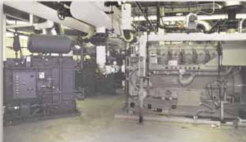
HOSPITAL , Chicago, Illinois (3) Model ESG1-616B18CSS. Recovering Btu from (3) Waukesha 3516, 1,100kW natural gas engines. Reducing each 2,392 SCFM from 1,135°F to 438°F. Delivering 2,173 pph steam @ 130 PSI operating (150 PSIG design).
