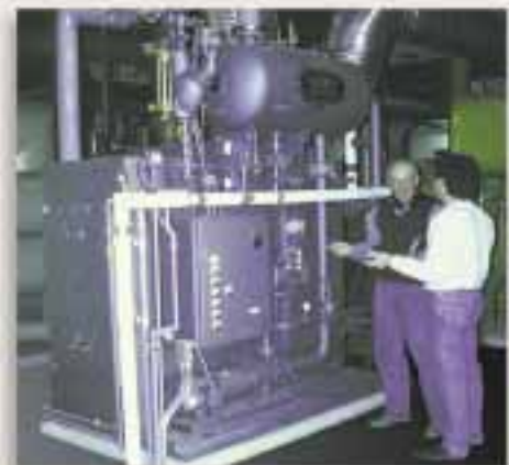
Field startup and operator training is realized quickly with factory trained personnel.
