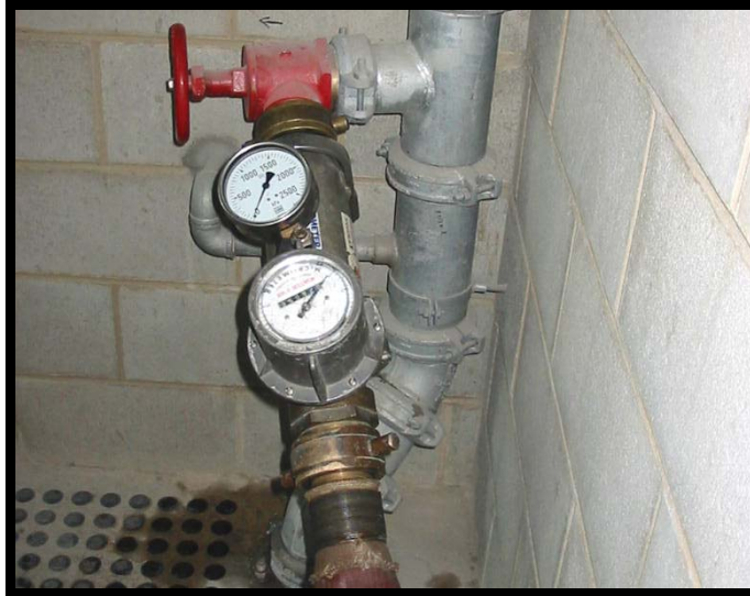
Figure 4 – Typical Observed McCrometer Test Arrangement
