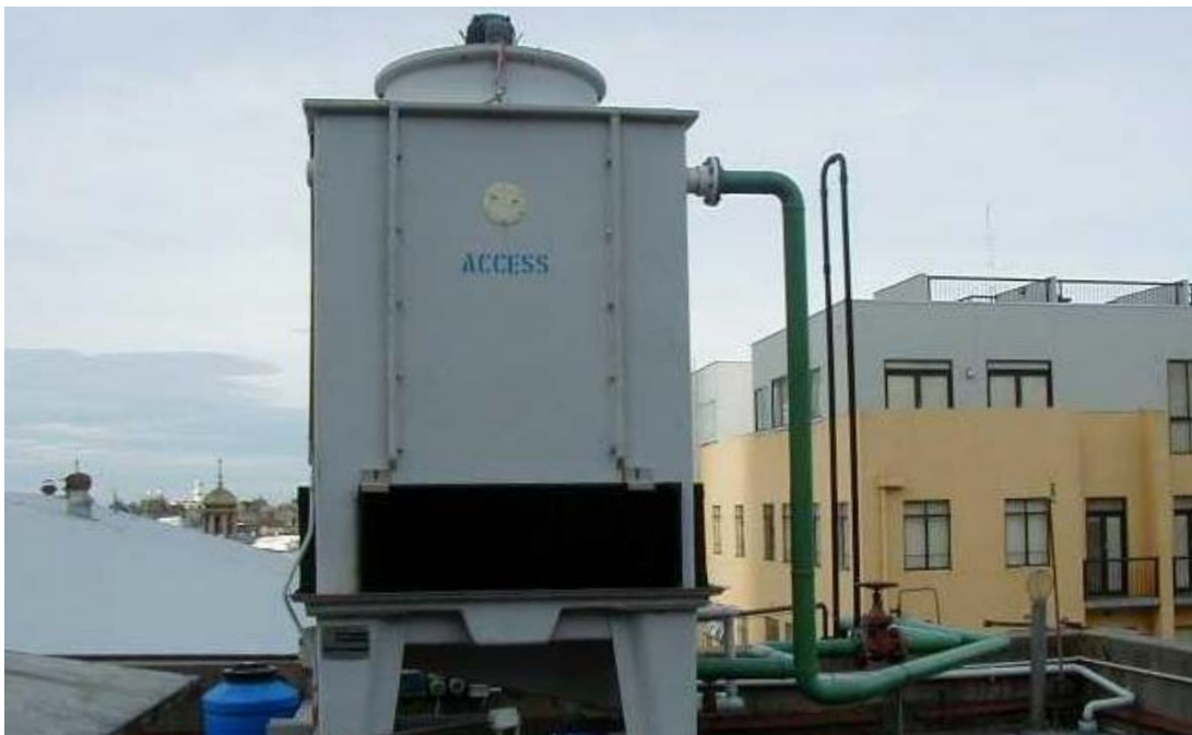
Changing risks: The re-development of an adjacent building to residential use has increased the numbers of people who live close to the cooling tower
