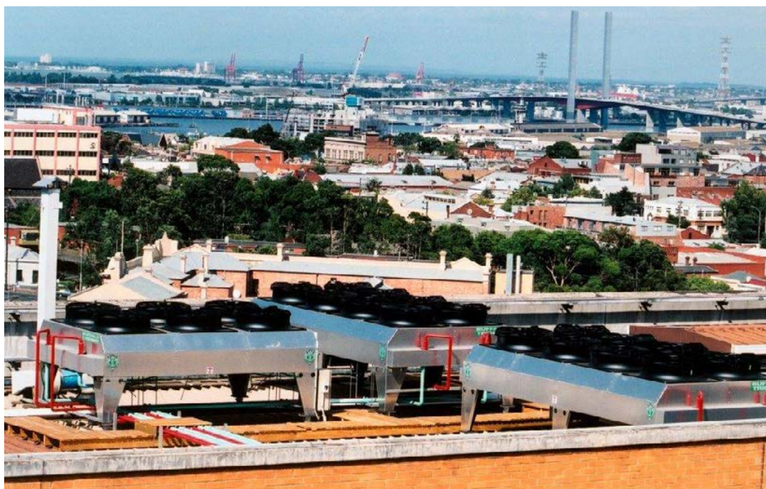
Air cooled system: Three air cooled systems forming part of an air conditioning system
