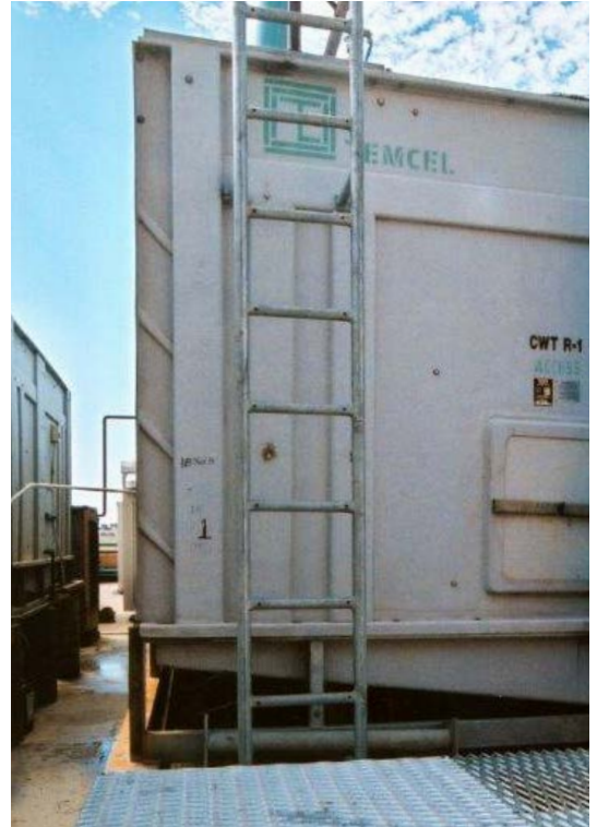
Tower ladder: Tower safety is important. Proper decking and ladders must be provided
