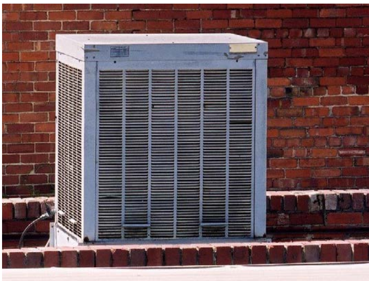
Evaporative Cooler: These units have not been linked to cases of Legionnaires' disease
