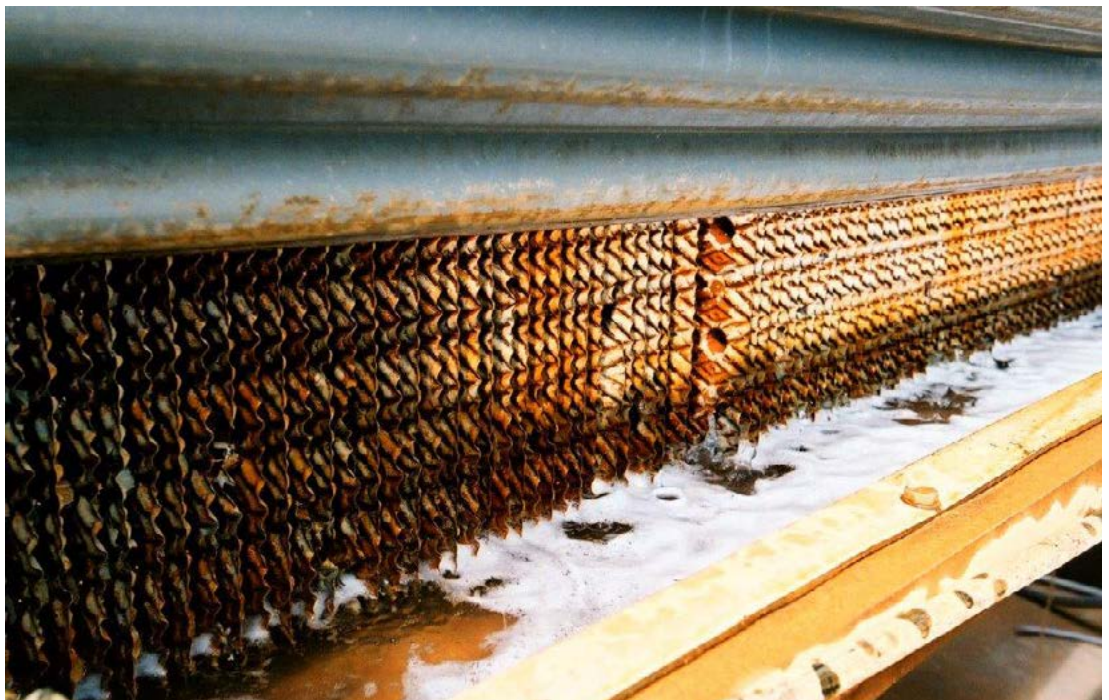
Cooling tower with basin exposed to sunlight: This cooling tower does not have sunlight protection to the side and basin of the tower
