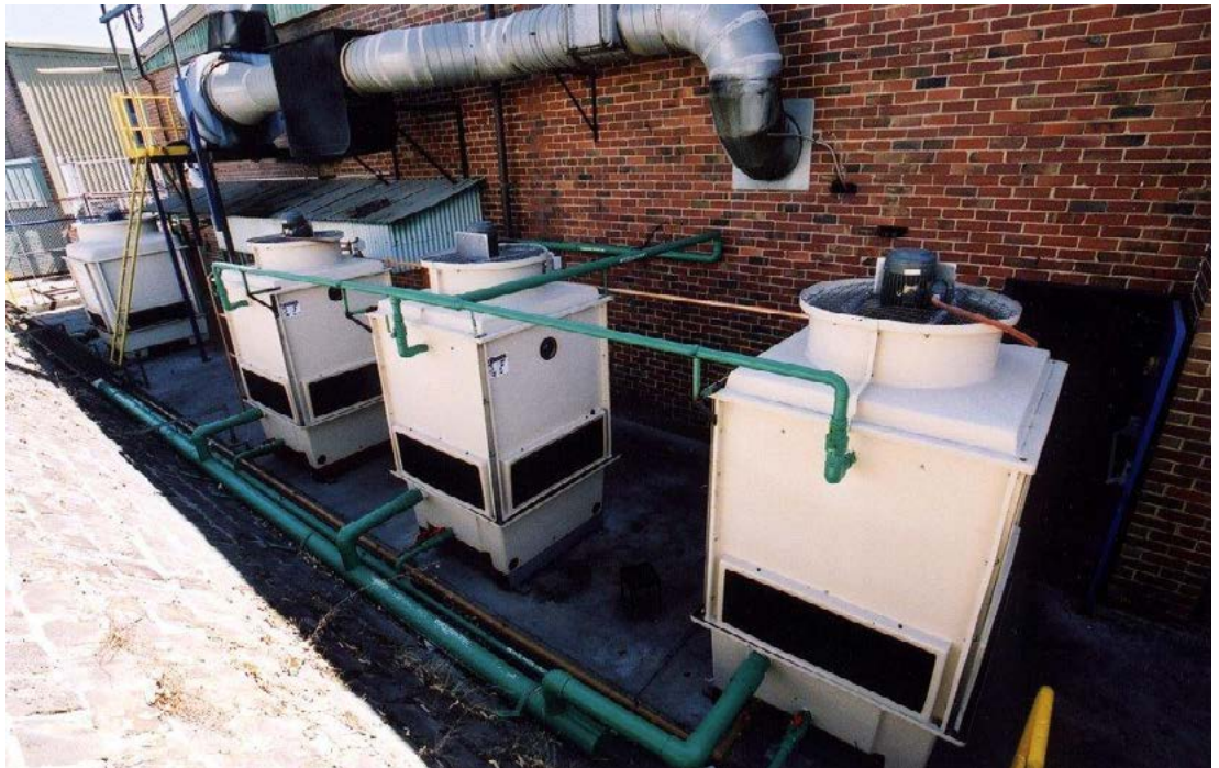
Cooling tower system: A series of inter-connected cooling towers that form part of a cooling tower system.
