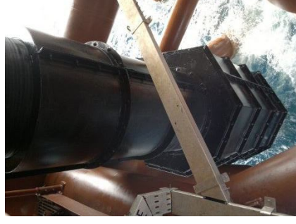
SS enclosure for riser anchor flange & pipe
