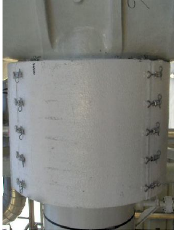
Epoxy PFP box on flange
