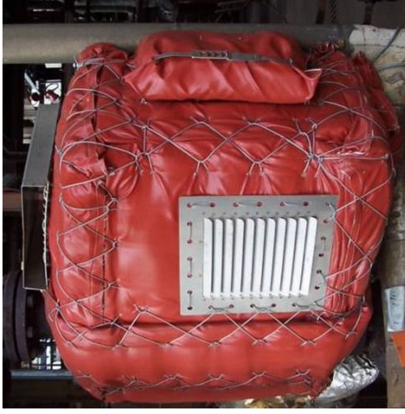
Ventilation grills for cooling and gas release
