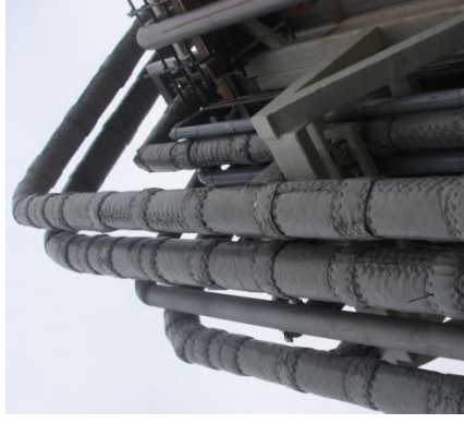
Flexible PFP jacket on piping
