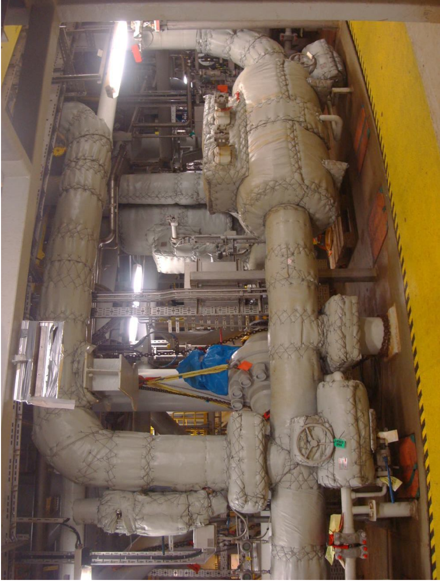
Jetfire PFP jackets installed on an FPSO turret riser sections
