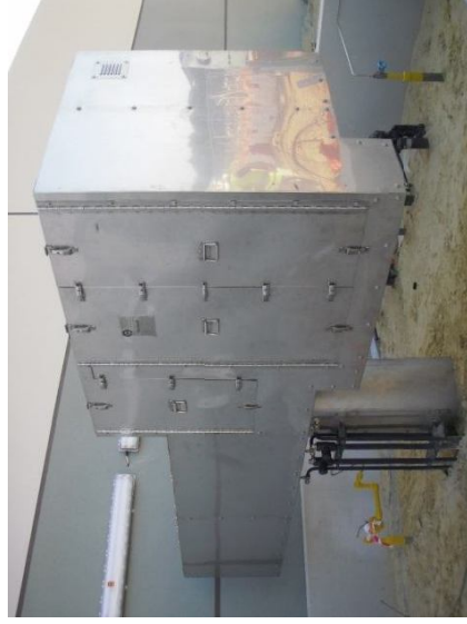
SS enclosure for actuator and controls
