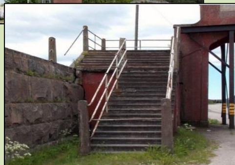
The Emigrant's Bridge is slated to be torn down next year to make way for expansion of the port.
