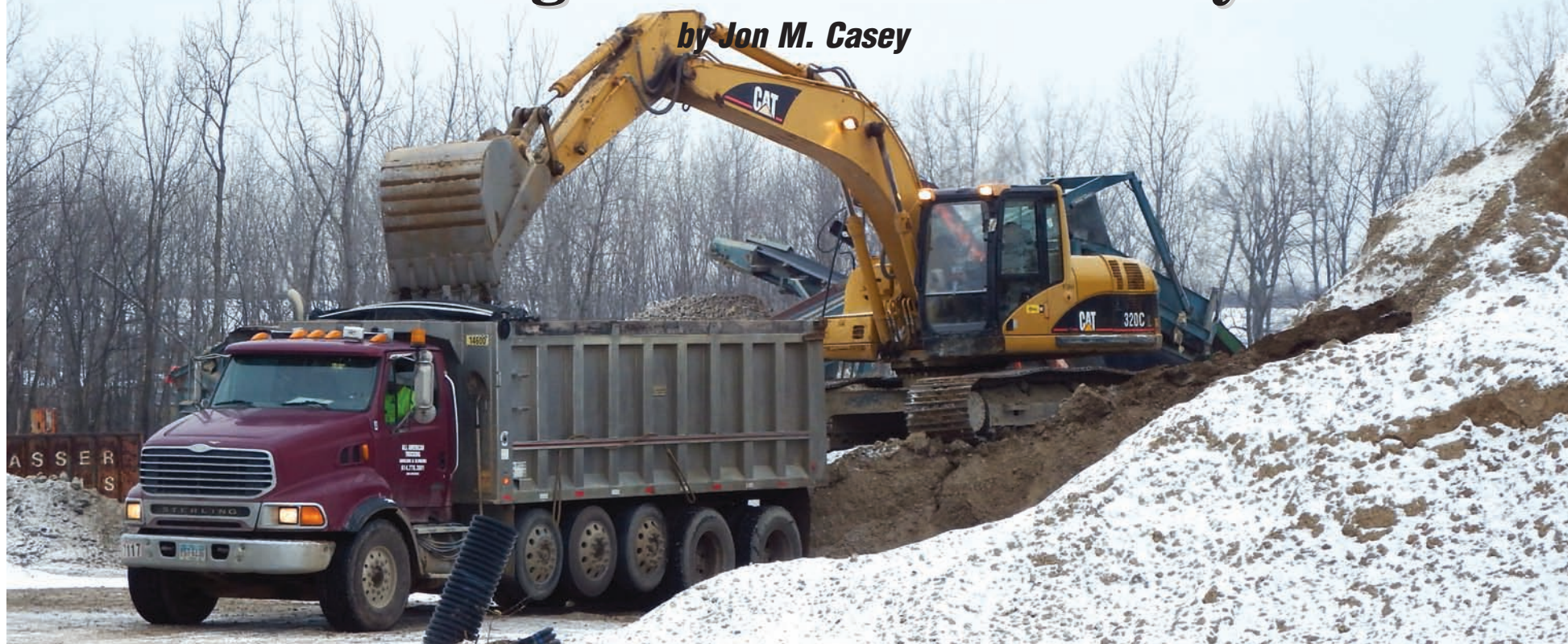
A load of 304s is headed out as Tom Clark fills an All American Trucking dump truck with material.
