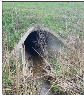
An existing 60" culvert under I-196 is the outlet for the Casco Drain
