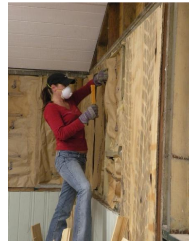
2LT Carla Mercier, 682nd Engineer Battalion, Minnesota National Guard, installs insulation in the Museum's workshop.
