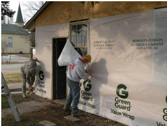
ECCC students place house wrap on a WW2 building before installing the outer siding.
