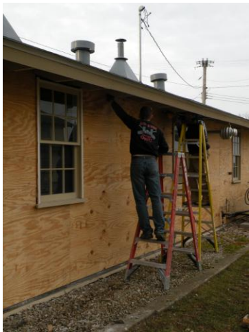
ECCC student placing sheathing on building 1318 which houses latrines for the WW2 area and the Museum's workshop.
