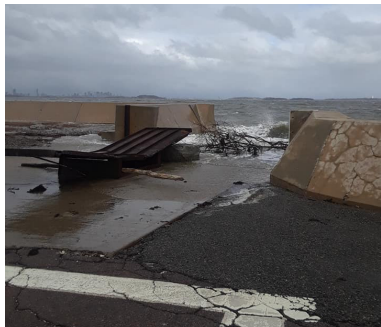
Damaged Sea Wall at Perry Beach
