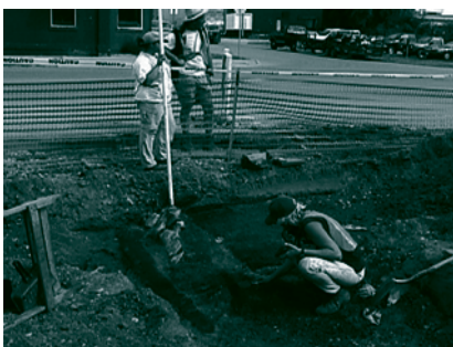
Staff archaeologists from the Louis Berger Group work to expose the foundation of an early structure along Third Street.
