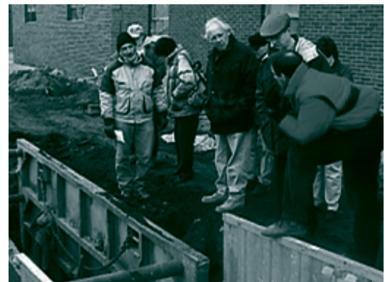
Chris Schoen, Marianne Long, Victor Roubidoux, Jeb Brewer, and Gene Schmitt inspect a deep trench excavation that required supports to prevent cave-ins.
