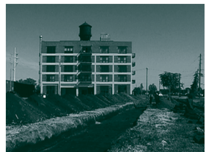
Looking down the excavated length of a utility trench along Martin Luther King, Jr. Parkway Portions of the enlisted men's cabins of Raccoon Row were exposed here.
