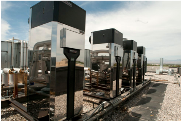
Four Camus DynaForce condensing boilers (outdoor) domestic water heating.
