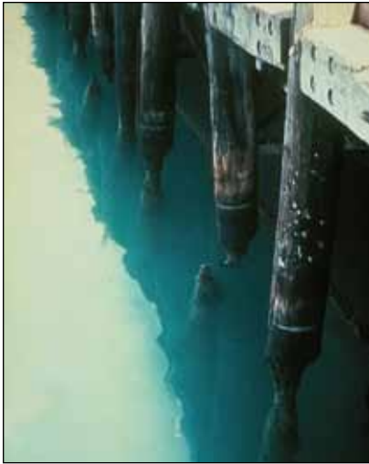
Figure 14–11. Limnoria damage to piling.
