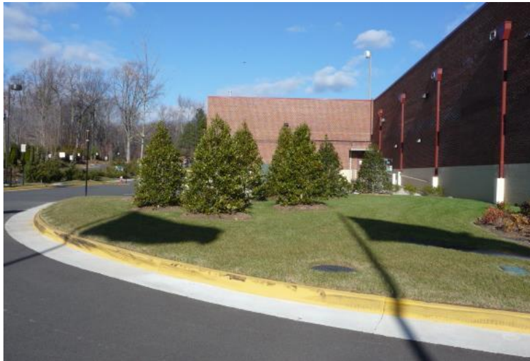
Figure 1216-C: The above image illustrates a vegetative screen that hides HVAC equipment and a dumpster.
