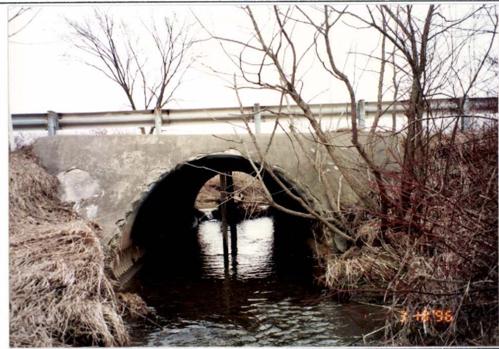
LOOKING @ LEFT SIDE OUTLET
