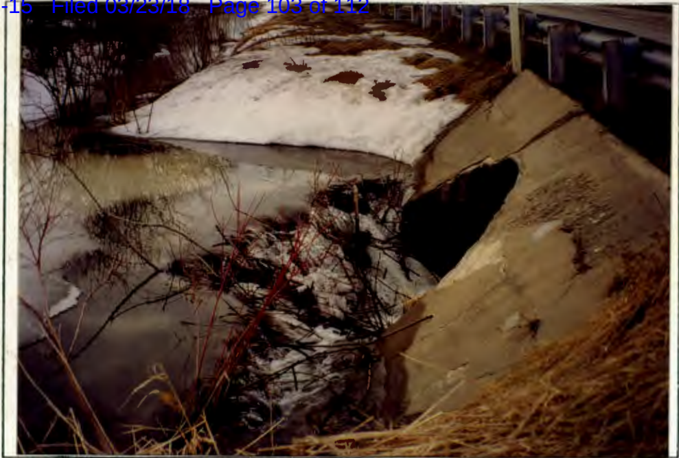
BEAVER DAM BLOCKING INLET
