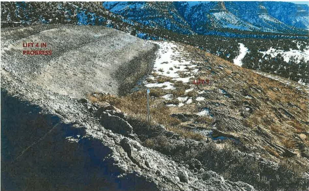
SCA#2 Ash Landfill – west face looking southerly Lift #3 covered and seeded. Lift #4 in progress
