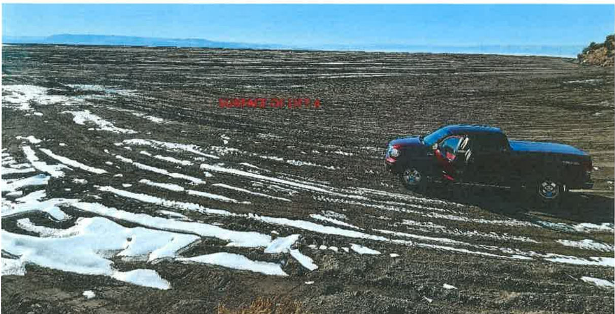
Surface of Lift #4 in process – photo looking northwesterly Compaction appears satisfactory. Dust suppression appears satisfactory Surface slopes east towards the hill to prevent storm water run-on
