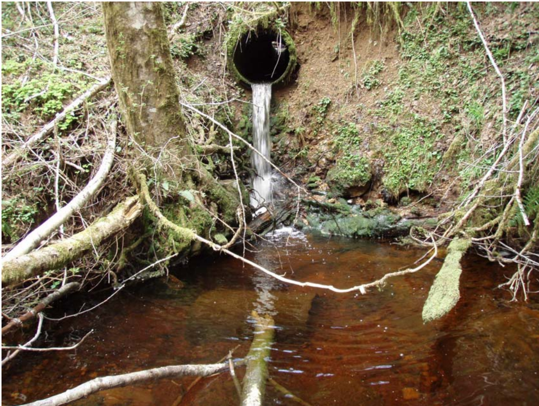
Figure 3.44. Photograph looking upstream at total barrier culvert in an unnamed tributary to Last Creek.
