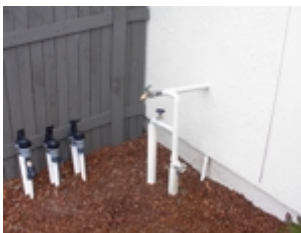
Photo 1 – Hose-bib and piping
