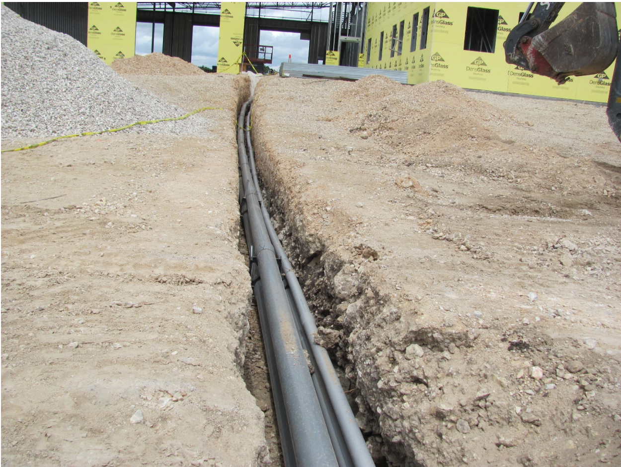
EXHIBIT 6 – MAIN ELECTRIC LINE 06.28.21
