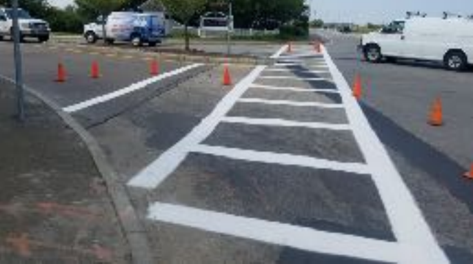
At E. Squantum St. & Victory Road all new striping after manhole repair
