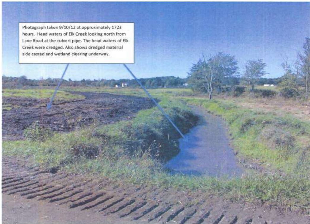
Figure 14. September 2012 photograph from Marsh Site inspection by Smolko; Elk Creek from Lane Road looking downstream (north) showing disturbed soils and side-casting from dredging Elk Creek.
