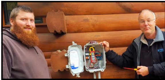
John Sheehan and Joe McDowell take a look inside the control box of a resident's sewer pump
