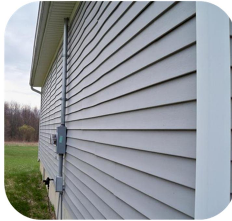
Imperfections in the wall can show through unsupported siding, giving your home a wavy appearance.
