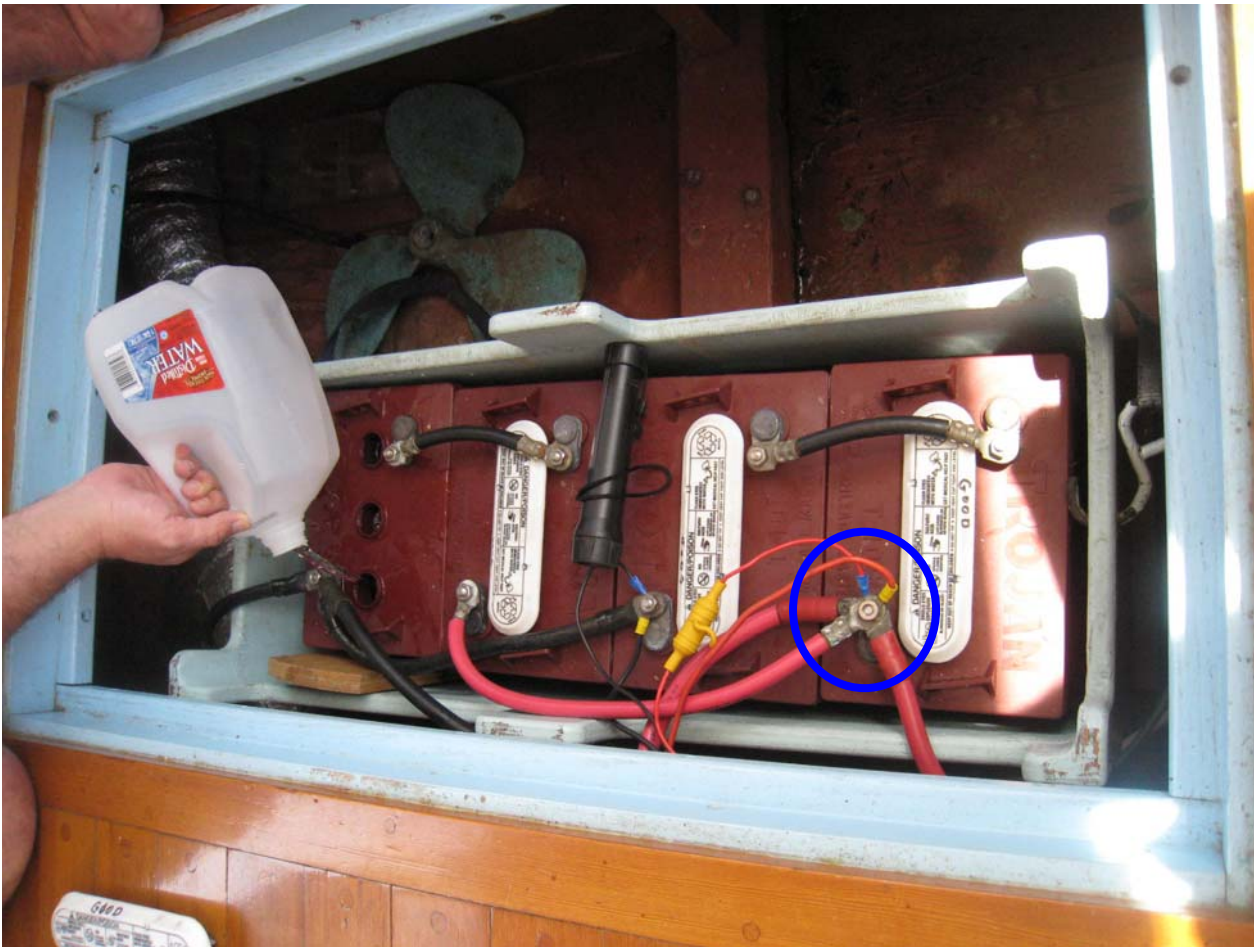
House battery bank being topped off with water. Per ABYC E-11. No more than four (4) terminals shall be mounted to a single battery stud.
