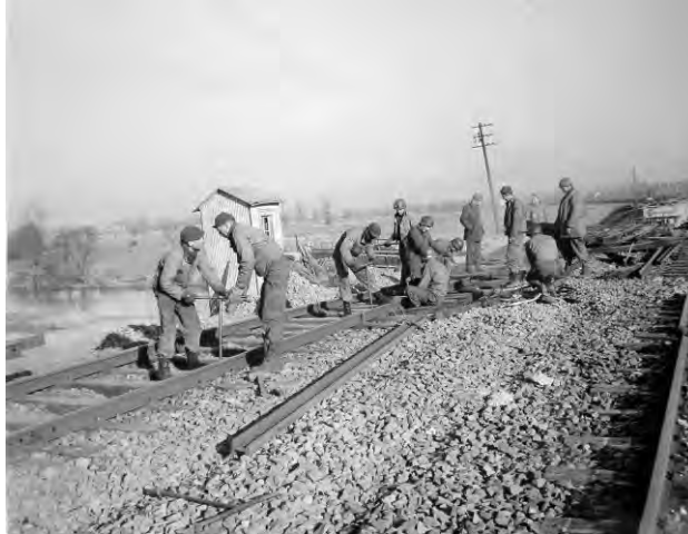
347 th Engineer Regiment Soldiers work to repair tracks destroyed by retreating Germans in Sarralbe, France—28 December 1944.
