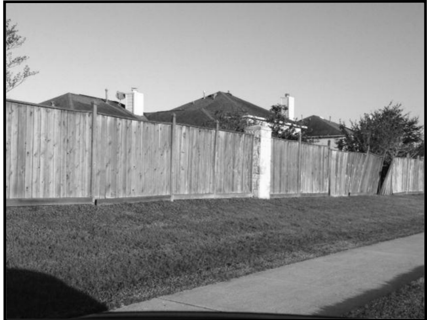
This is the Burney fence which is still in need of repair!
