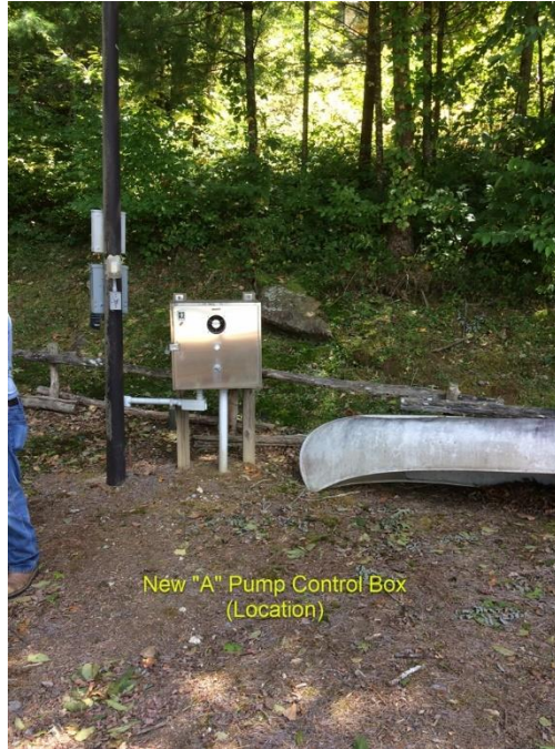
Image: “New A” Well Pump control box
