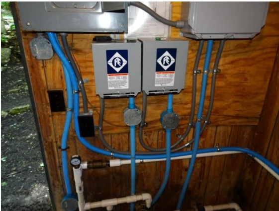
Image: Piping below control boxes
