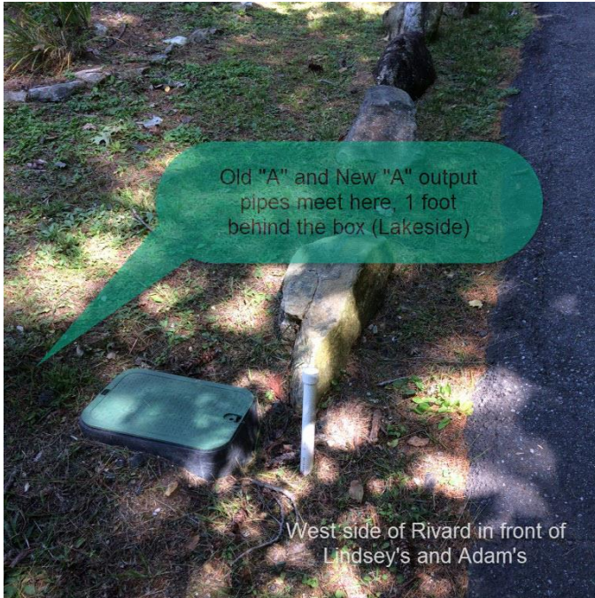
Image – Junction Box on Rivard
