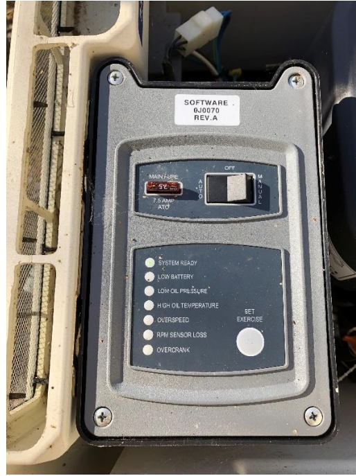
Image: Status Panel Enlarged. Note 7.5 Amp Auto Fuse. ,
