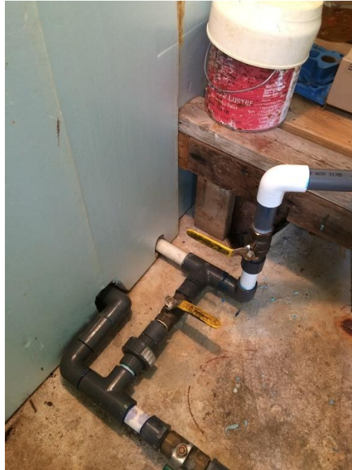
Image: Closeup of Crossover Valves (Redo this pic)
