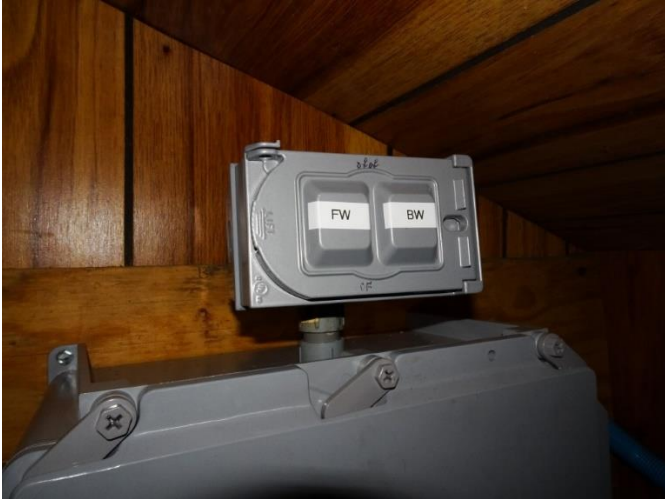
Image: South Well control house Well Selector Switch
