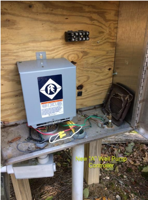
Image: Inside "New A" Well Pump Control box
