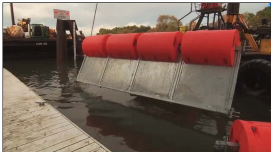
Figure 31. Floating wall being installed near the entrance to Georgiana Slough in 2014 (screen capture from: http://www.youtube.com/watch?v=937bXx9QMn8&feature=youtu.be )
