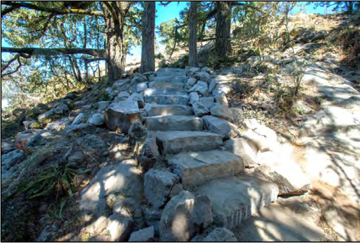
Constructed stone steps on a steep section of trail on Spencer Butte in Eugene
