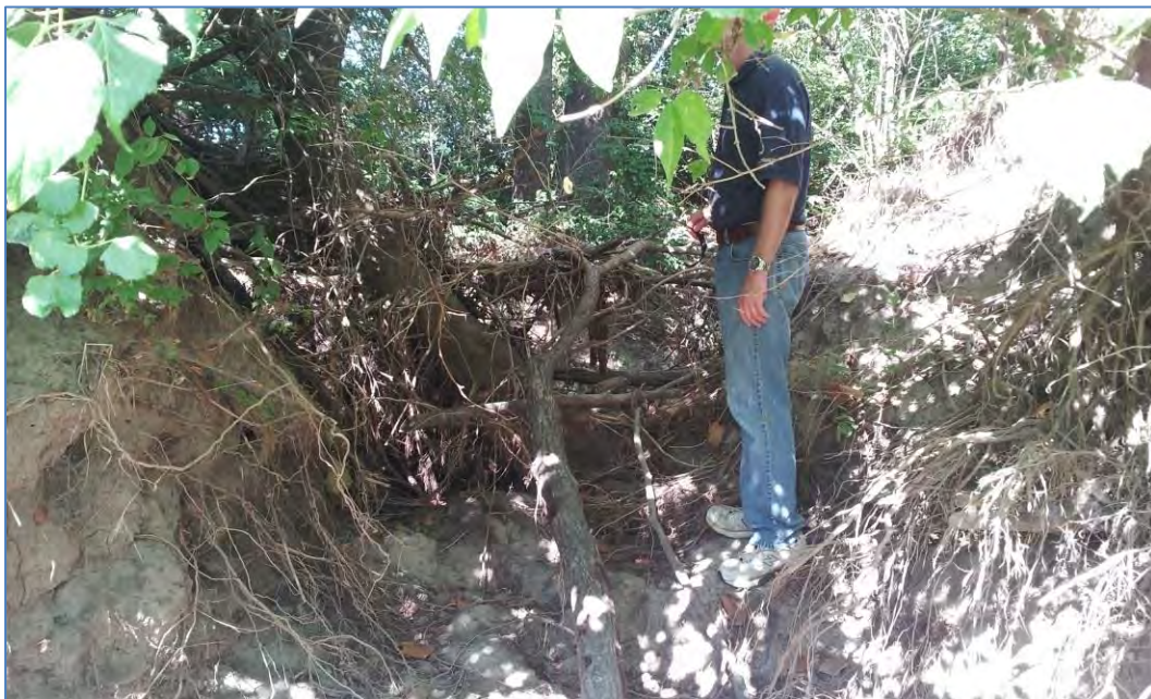
Figure 4-23: Breach in Berm at Offline Detention Area near Fourlakes Drive
