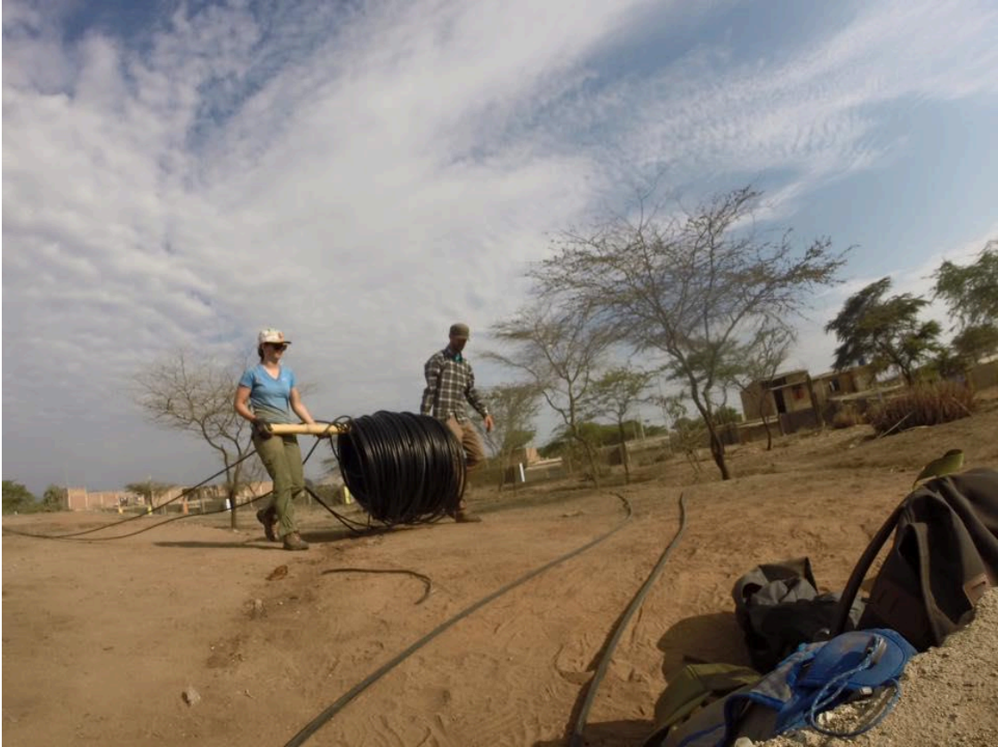
Installing an irrigation system to maintain a newly developing conservation park, in the harsh desert climate of Ferreñafe.
