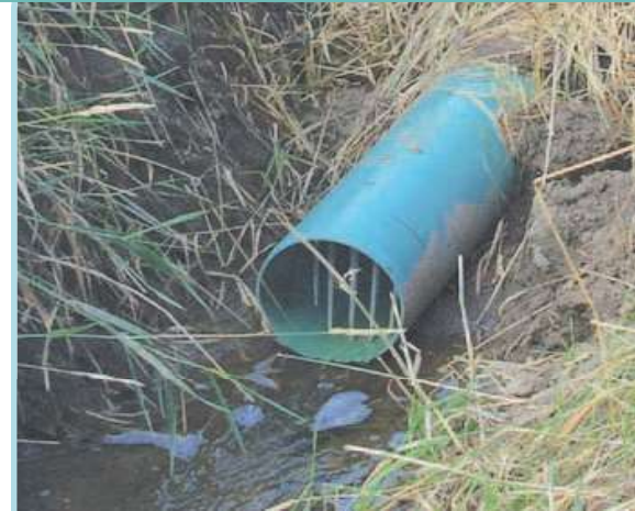
Figure 1: Tile outlet with a rodent guard.
