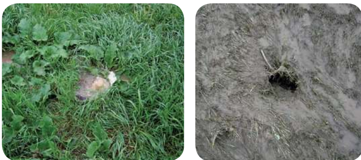
Figure 3: Sinkholes caused by tile blowout.
