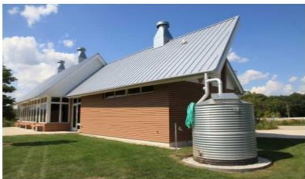
Figure 4: Rain Water Gutter System
