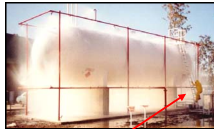
AMCOR plant – me checking system
