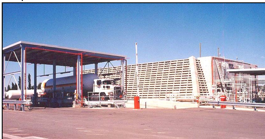
ELGAS distribution at Blacktown
