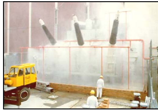
Wallerawang Power Station, Transformer protection
