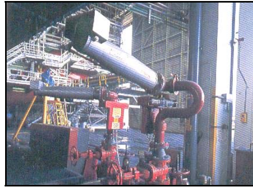
Fire equipment in the new hangar
