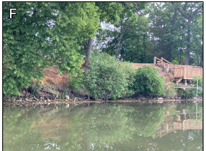
Photo 12. Undercut bank with exposed roots.
