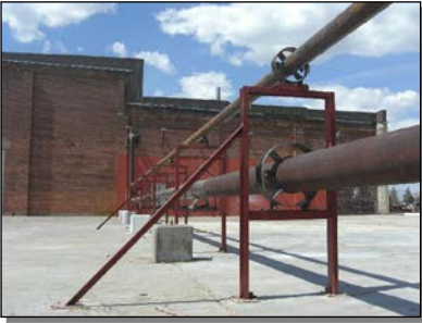
FAFB Building 2249 Steam Piping
