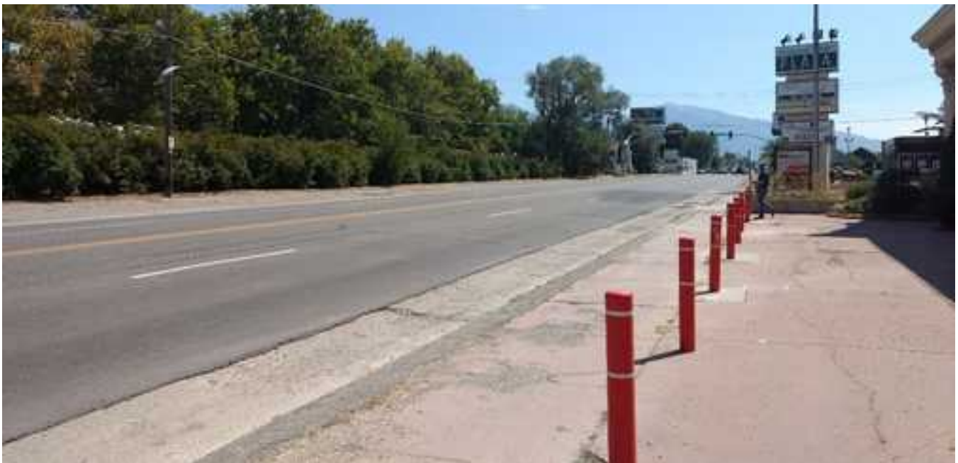
Rolled Curb and Poor Sidewalk Conditions on Highland Drive
