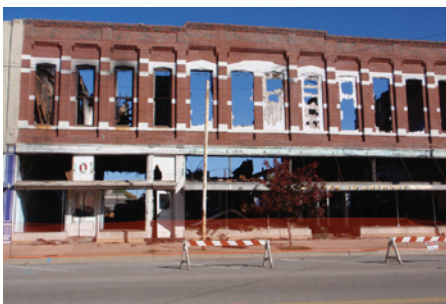
One of the facades of the burned buildings.
