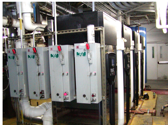
Four Camus DynaForce condensing boilers (indoor)– domestic water heating.
