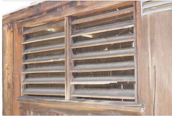
Figure 9: Pump House Ventilation – Western Exposure
