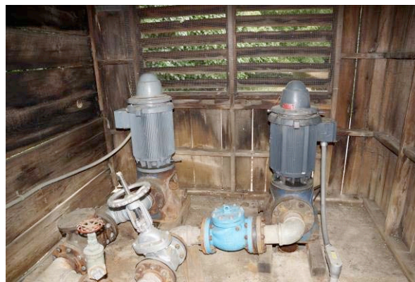
Figure 8: Pump Motors in Pump House
