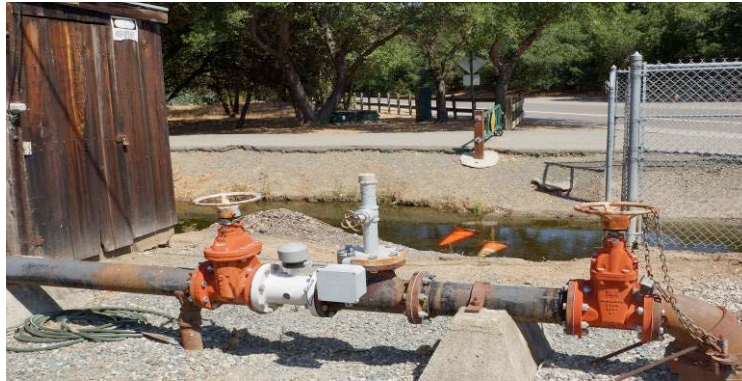
Figure 10: Discharge Header from Pump House
