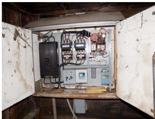
Figure 7: Pump Controls in Pump House
