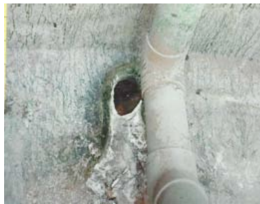
Figure 19: Tank Foot Valve, detail
