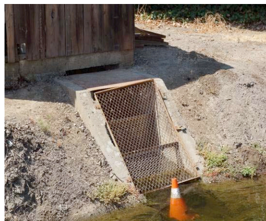
Figure 5: Pump Station Inlet Screen
