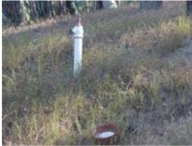
Figure 20: District Wharf Hydrant
