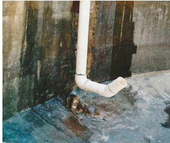
Figure 11: Raw Water Discharge Point
