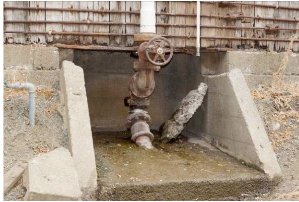
Figure 18: Tank Shut Off Valve and Fill Line
