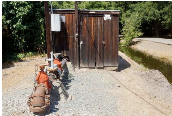
Figure 6: Pump House and Discharge Pipe
