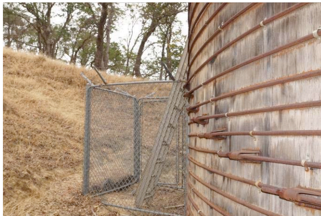
Figure 15: Tank Ladder Security Fencing
