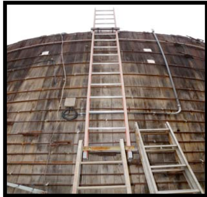
Figure 13: Tank Access Ladder, Ext.
