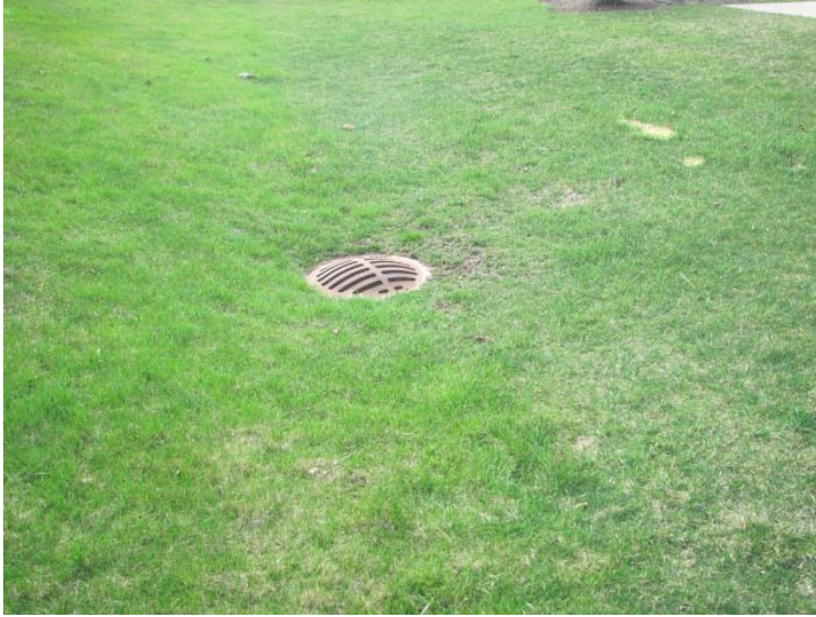
Typical landscape catch basin
