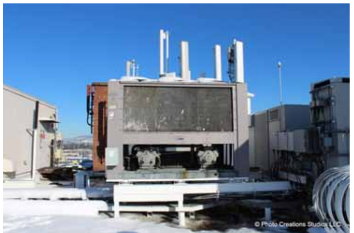
ROOF – CHILLER & PUMPS
