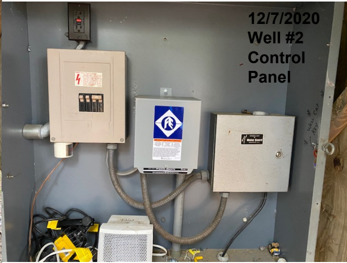
12/7/2020 Well #2 Control Panel
