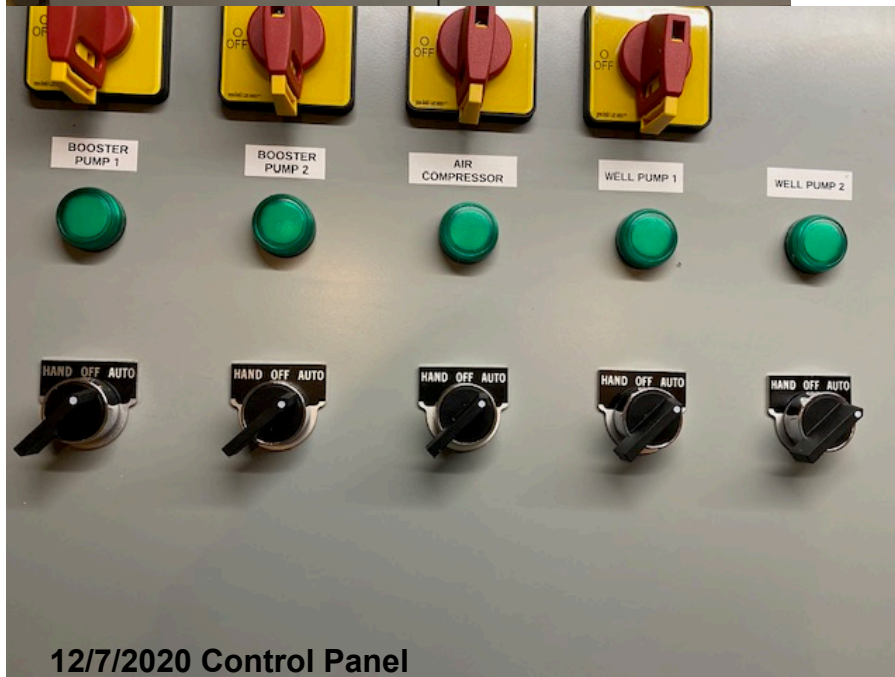
12/7/2020 Control Panel in Treatment Building
