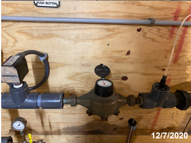
12/7/2020 Raw Water Isolation Valve
