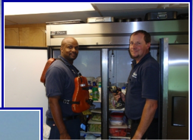
Techicians David Smith and Steve Phillips install a new drain pan in the cooler.
